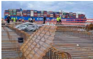
Onshore LNG Terminal in Stade, Germany
